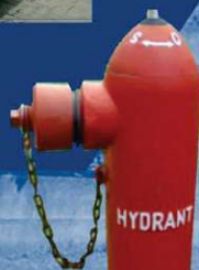
HIDRANT PEMADAM KEBAKARAN Hydrant Firefighter
